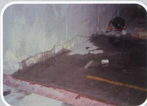
COLD JOINT REPAIR — BEFORE
